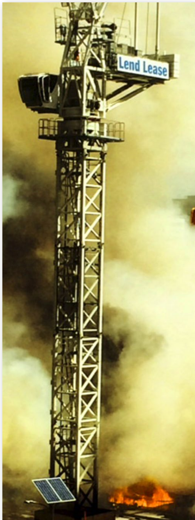
Fire at Sydney's largest building site, Barangaroo, on 12 March, 2014. Unfortunately evacuation procedures left a lot to be desired with over 100 workers unaccounted for hours after the alarm.
